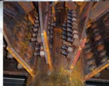
The Concert Hall's roof is supported by six 20-ton trusses arranged in a spoke formation, attached at a single connection point with more than 120 bolts. This is a close up of the connection of radial trusses to truss T9.
